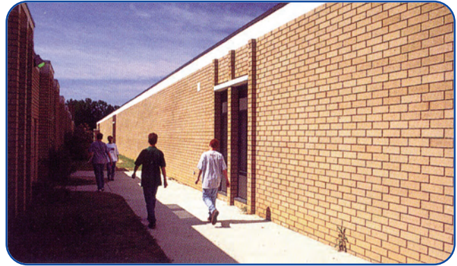
Students walk along North Augusta High School's new foreign language wing, which had a severe moisture problem five years after it was built.
